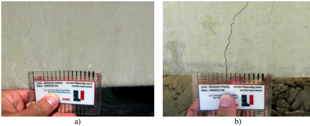
Figure 4. Cracking in the tensioned face of the stored piles due to their own weight: a) a steel reinforced pile; b) a GFRP reinforced pile.
