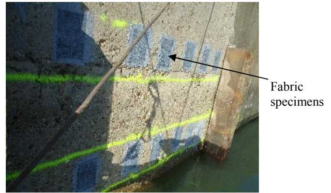
Figure 4: Bonded carbon fabric specimens on a quay wall in the marine environment
