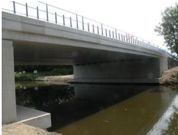
Figure 2. Traditional concrete edge elements installed on bridge Slootdorp N240 (picture Holland Scherm)
