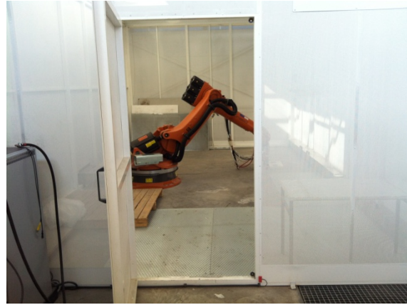
Figure 2.- Isolated cell with 6 axis robot and magnetron
