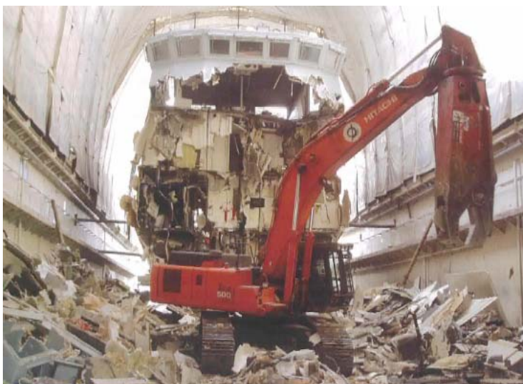
Figure 10: Scrapping of a 55 m composite sandwich hull with an excavator with hydraulic jaws
